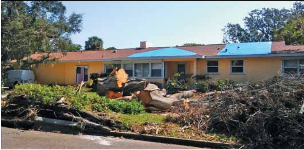
Tree and roof damage caused by Hurricane Irma. Recorded gusts in the St. Petersburg area ranged from 69mph at Albert Whitted Airport to 92mph in the vicinity of Fort De Soto. Courtesy of Michaels Family Collection
