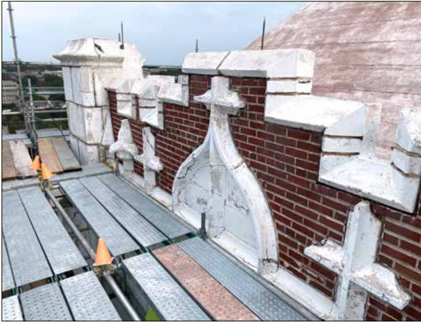
Church concrete ornamentation in need of repair
